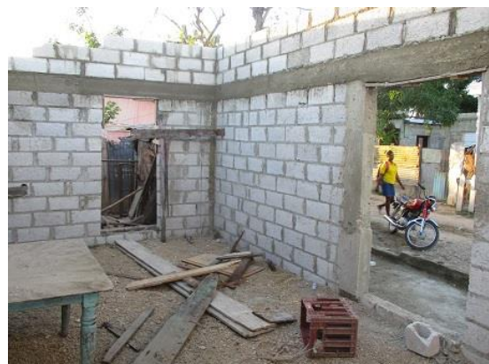
Roughly the same view after the stabilizing layer was finished and the staggered blocks in place for the roof incline.
