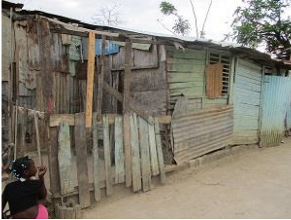
Avida's house before the construction ministry got involved.
