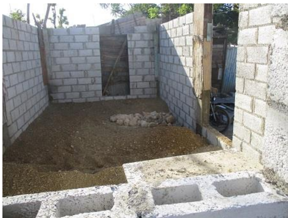
The columns have been poured and they are putting in the filler for the floor.
