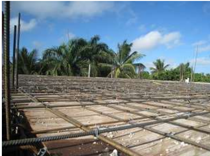
Rebar in place in summer 2013, ready for the roof to be poured.
